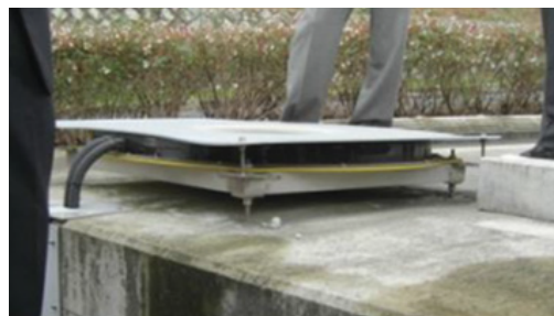
Fig 1.2: The Deployed Tx Coil of the Stationary Charging System at Bus Stops, Deployed in Waseda University, Japan [5]
